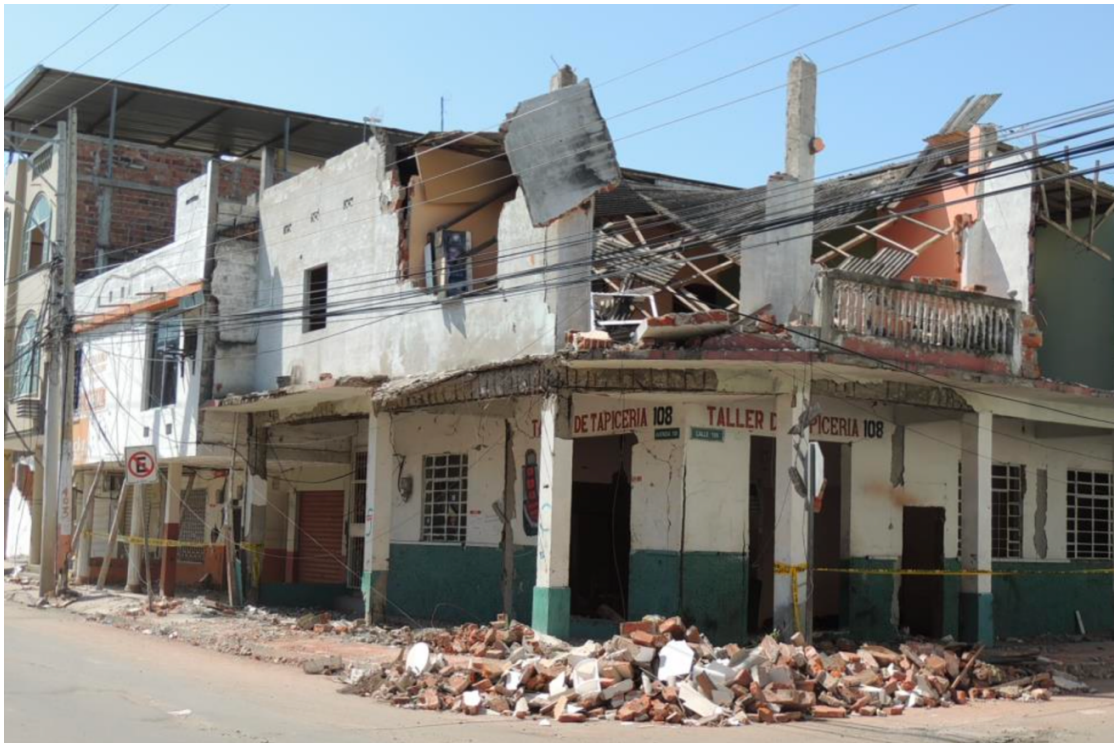
Fig. 7. Residential building in Tarqui, Manta, where the exterior walls collapsed. The roof also fell in this property. Adapted from Nicolaou et al. 2016.
