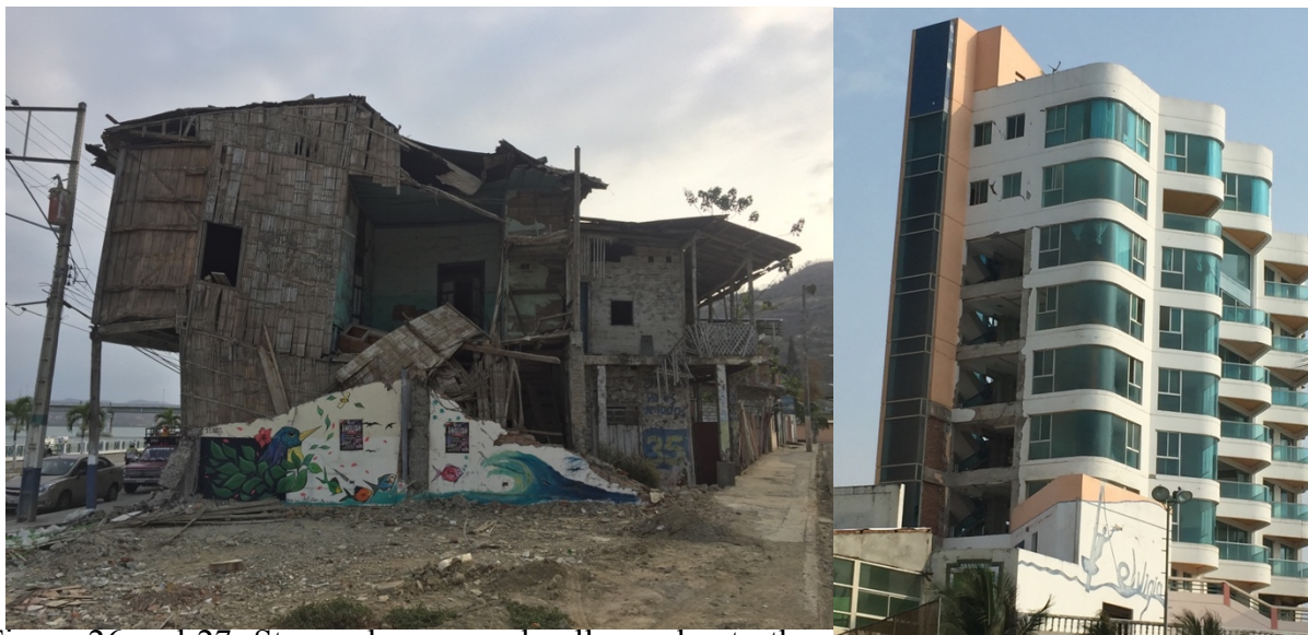
Figure 26 and 27: Strong damage and collapse due to the earthquake of Muisne in April 10, 2016, close to the entrance to the city of Bahía de Caráquez, as well as in the hotel area.
