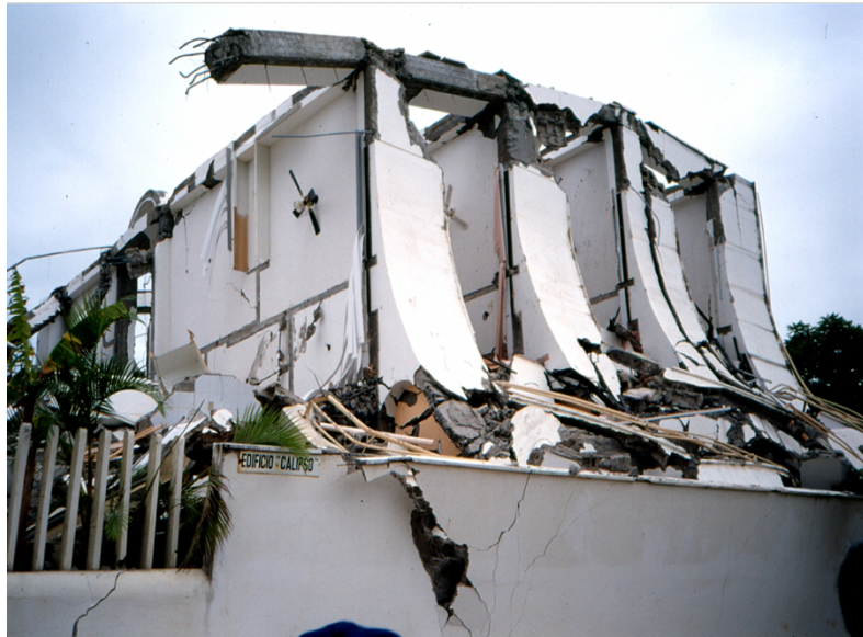
Figure 25: Collapse of the hotel Calypso due to the earthquake with an epicenter close to Bahía de Caráquez on the August, 4 in 1998.
